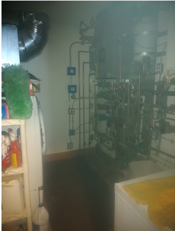
laundry in hydronic heating room off of kitchen
